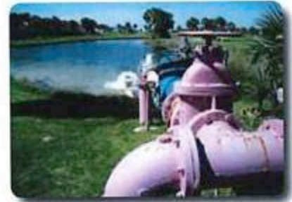
In the United States and other countries, purple pipes are used to distinguish nonpotable distribution systems, helping to prevent cross-connections.
