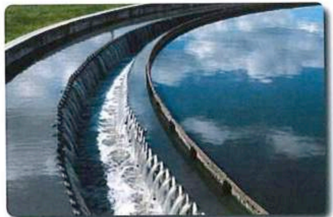
Secondary sedimentation basin in a wastewater treatment plant.
